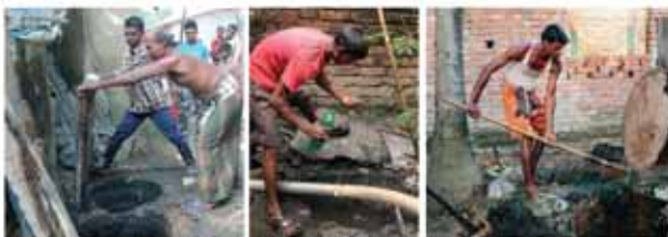
Work without personal protective equipment
