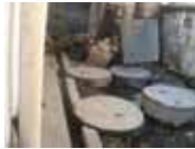
Overflow of septic pit
